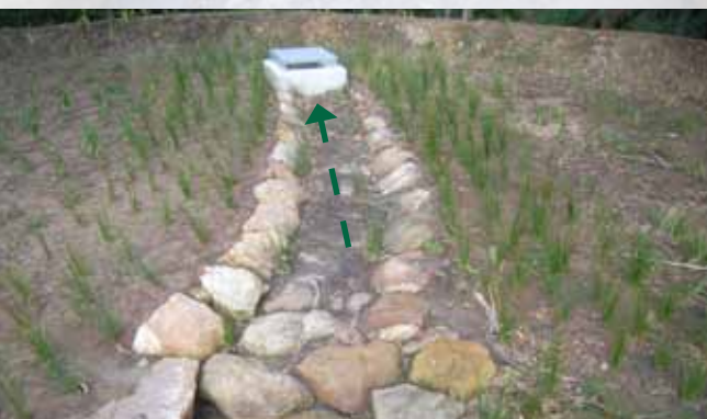
Rock lined inlet to leaf collection pit on Denman Avenue
