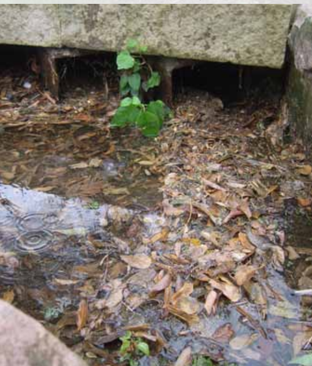
Stormwater inlet points into rock sedimentation basin (there is a large amount of leaf debris in the basin after a recent storm event).
