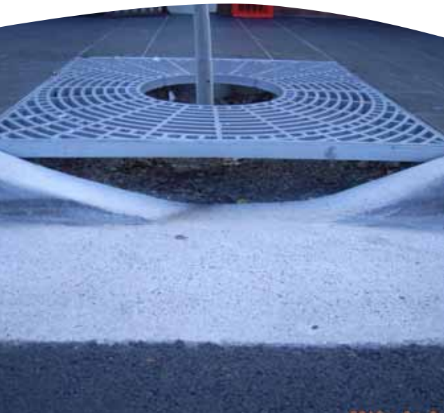
Inlet to one of the biofiltration tree pits along Railway Road
