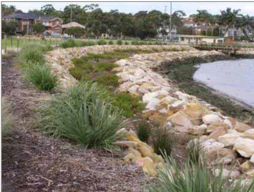
Figure 4-17. Intertidal saltmarsh area between rock sills, and upland riparian groundcover (Claydon Reserve, Kogarah LGA)
