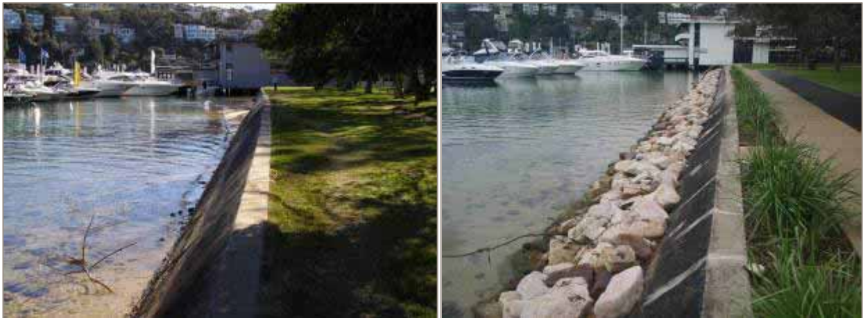
Figure 4-16. Incorporation of various sized rock boulders at toe of seawall Pearl Bay, Mosman LGA
