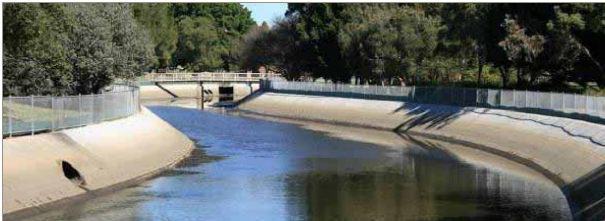
Figure 4-9. Concrete lined canal with steel fence along crest to prevent public access
