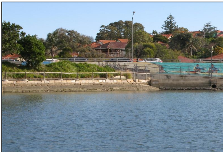
Photo 1 Sloping and vertical sandstone blocks and concrete sea stairs sections of the seawall.
