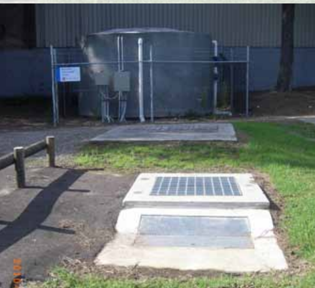
Stormwater inlets and 30kL tank
